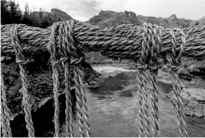
An up close example of the braiding techniques used to create the materials for the bridge.
